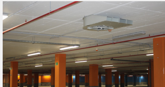
CAR PARK VENTILATION Madrid RIO shopping centre, Spain
