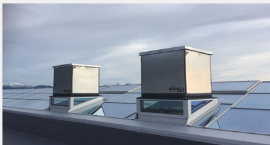
SMOKE EXHAUST Romsdal High School, Norway
