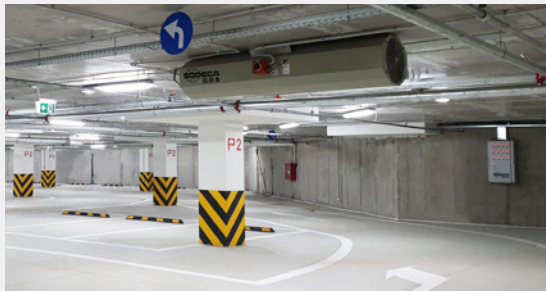
CAR PARK VENTILATION Hotel Sheraton Grand Tbilisi Palace, Georgia
