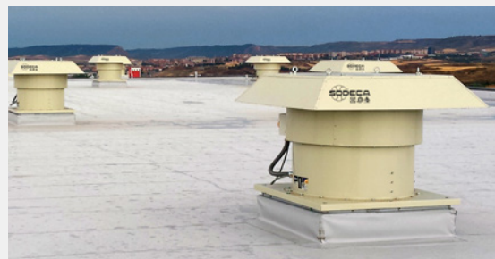
SMOKE EXHAUST Silo Inditex, Madrid
